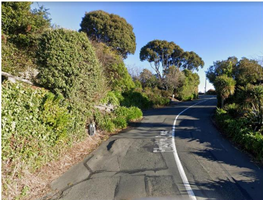
Figure 4: Fifeshire Crescent no footpath on either side of the road
